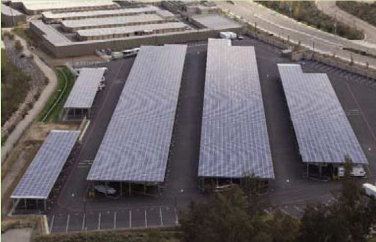
The panels atop Temescal Canyon Storage provide 1.75 MW of direct-current solar power.
